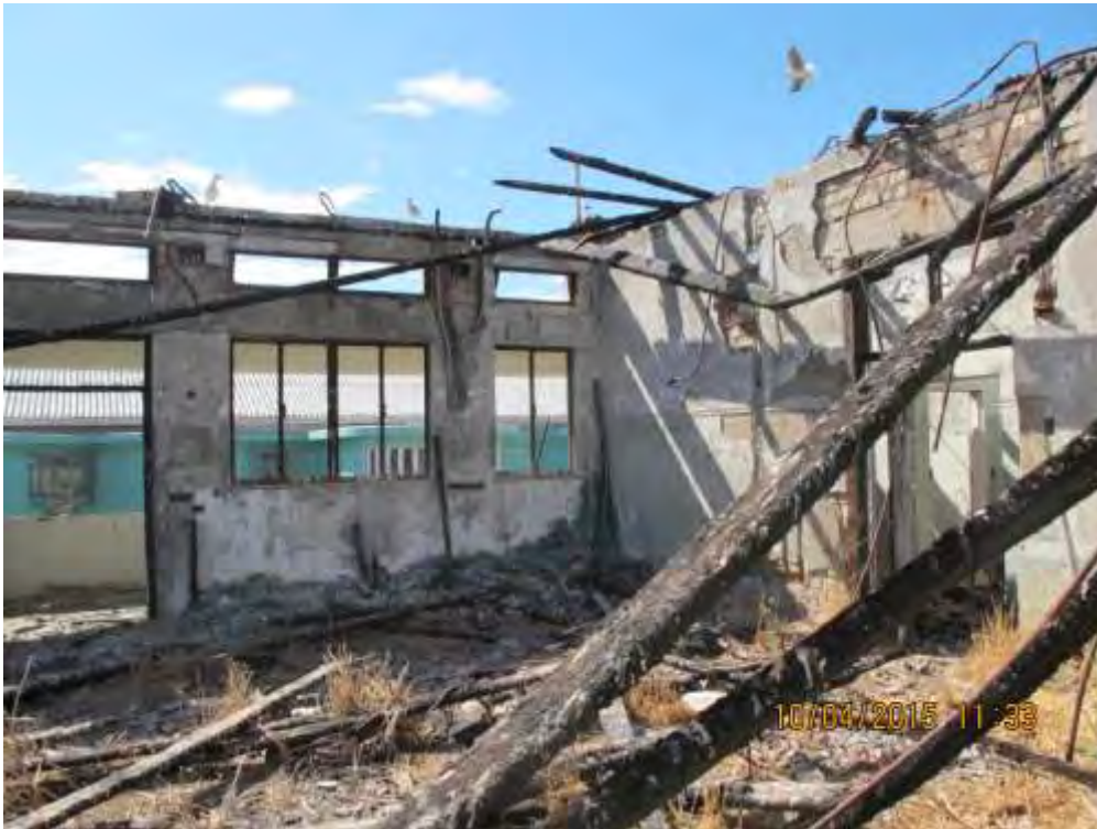
BUILDING 62 - FIRE DAMAGED
