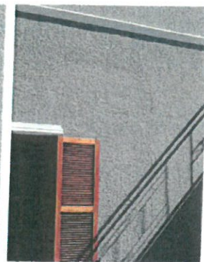
Evidence of old doorway
