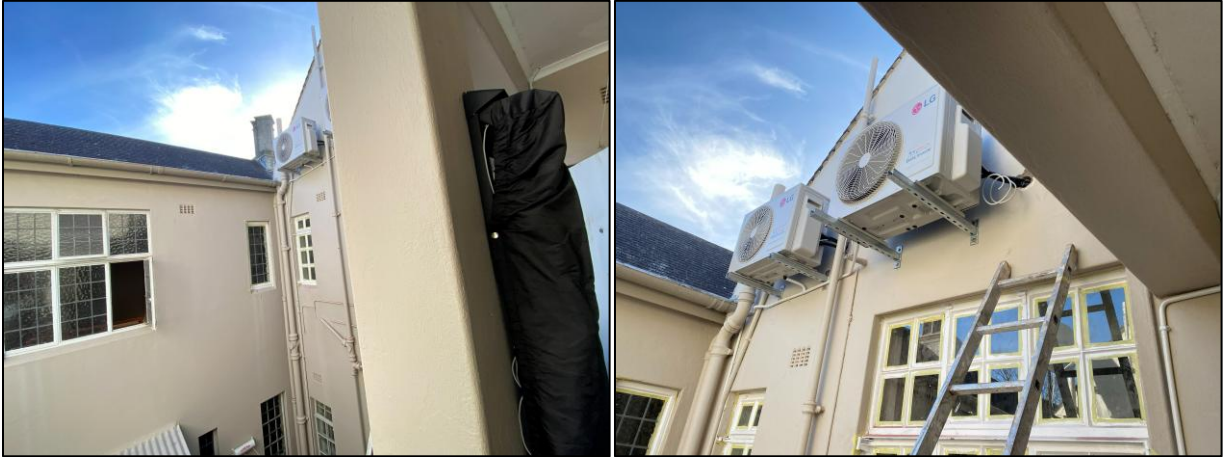
Figure 3. Aircon condenser location is within a shared internal courtyard area and is not visible from external views of the property.
